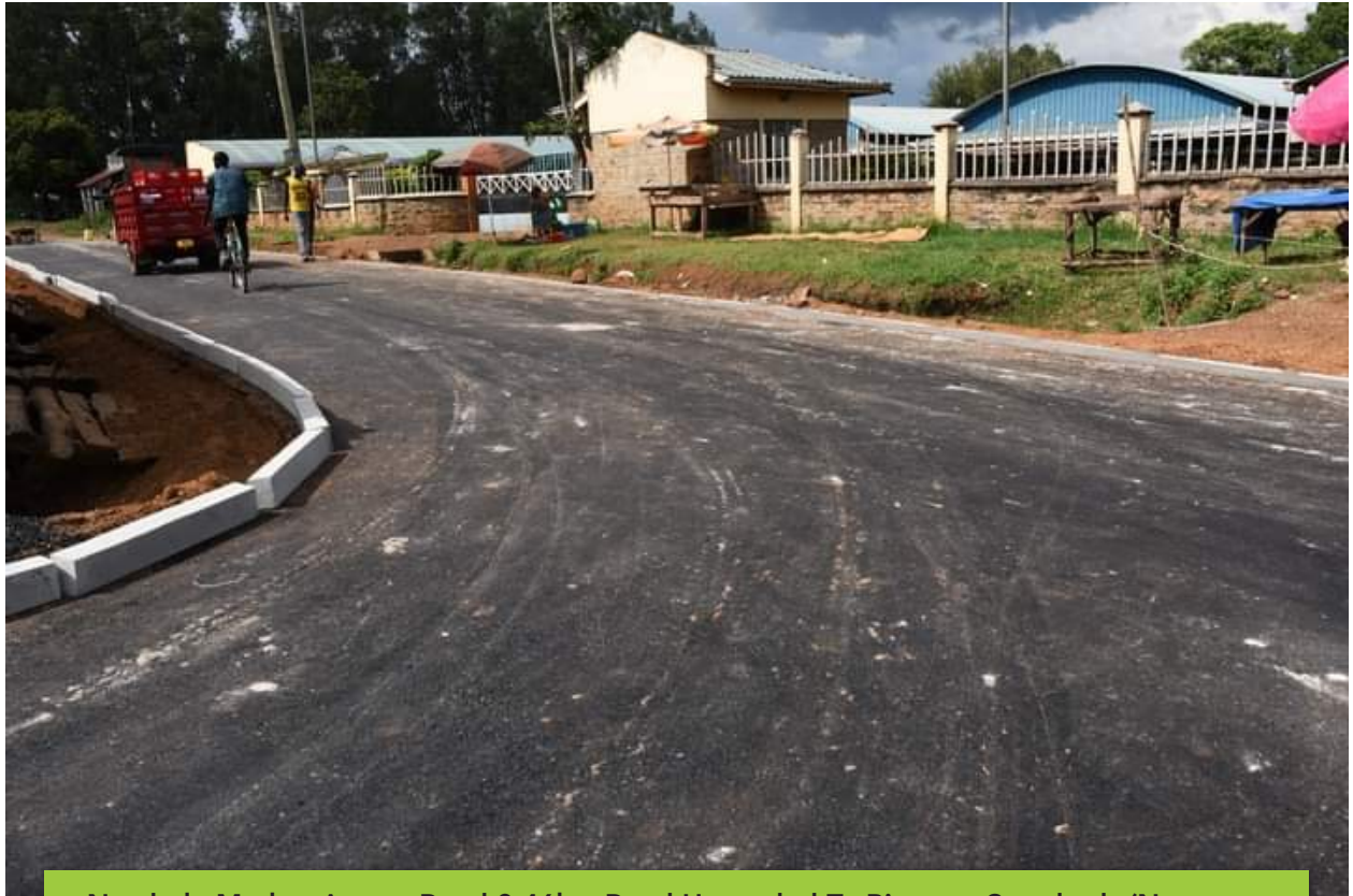
Nambale Market Access Road 0.46km Road Upgraded To Bitumen Standards (Nambale Sub –County)
